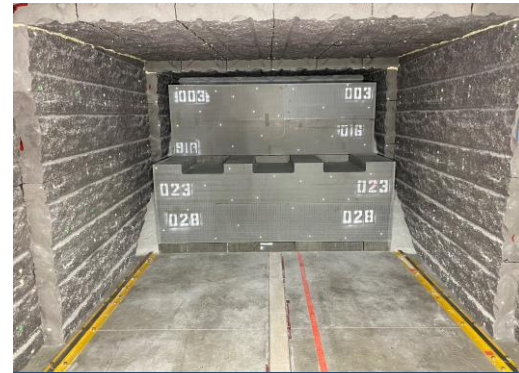
Full Scale Emplacement of EBS components in mock-up underground room (courtesy NWMO)
