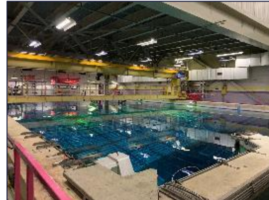
Pickering NGS Spent Fuel Bay
