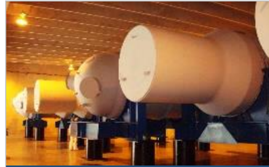
Bruce Power Units 1 & 2 Steam Generators
