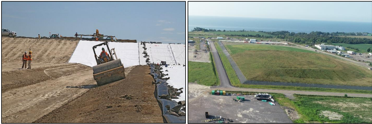
Figure 15: Installation of Liner (left) and Capped and Closed Facility (right) in Port Granby, Ontario
