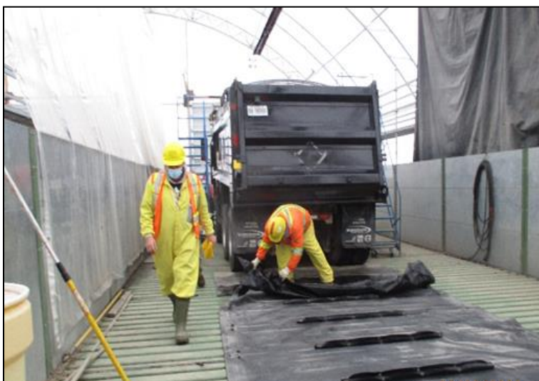
Figure 26: Performing Truck Inspection at the Monitoring and Decontamination Bay
