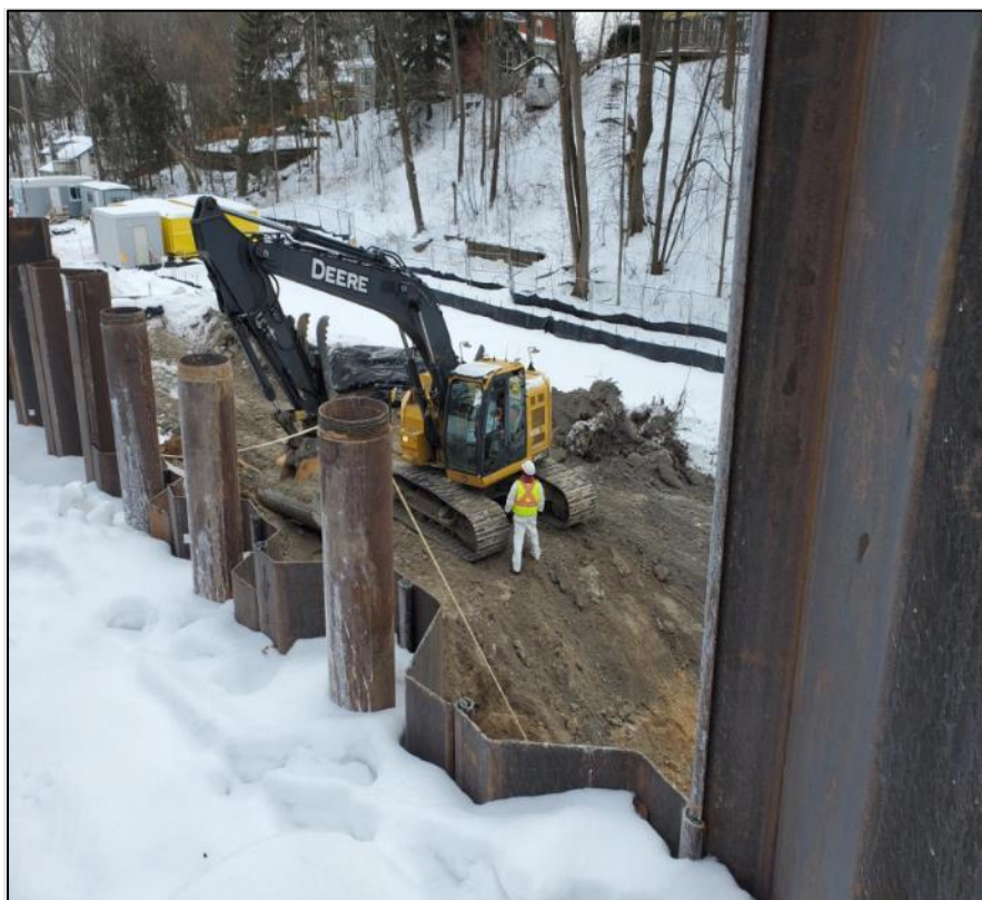
Figure 37: Strachan Street Ravine Waste Removal - February 2022
