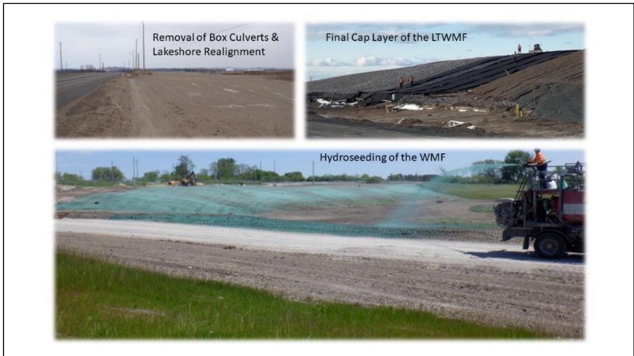
Figure 14: Final Construction Activities for the PG LTWMF and the former Waste Management Facility
