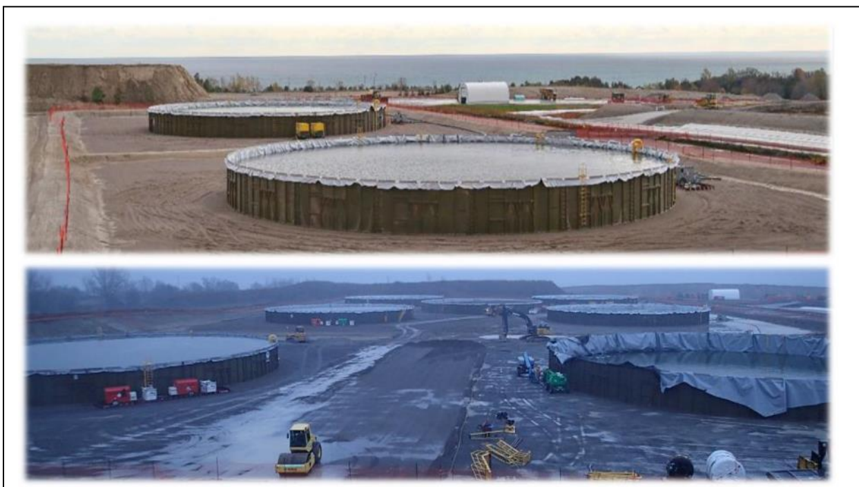
Figure 11: PG LTWMF Lake Tanks for Bulk Storage of Impacted Water
