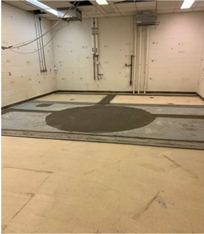
Figure 4-7: SRC pool and overflow channels filled with grout during decommissioning (Source: SRC)
