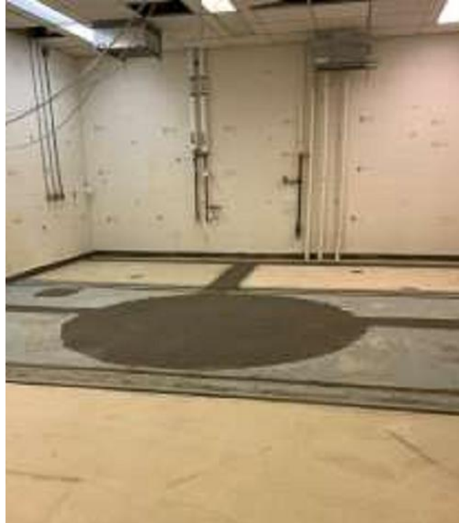
SRC Reactor Facility pool and overflow channels filled with grout Source: SRC
