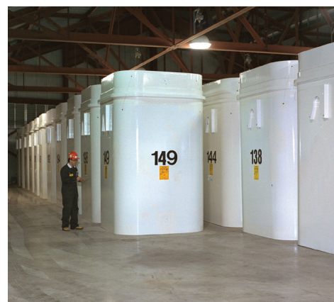
PWMF used nuclear fuel storage canisters
