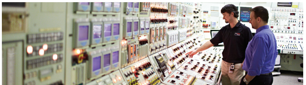
Pickering Nuclear Control Room
