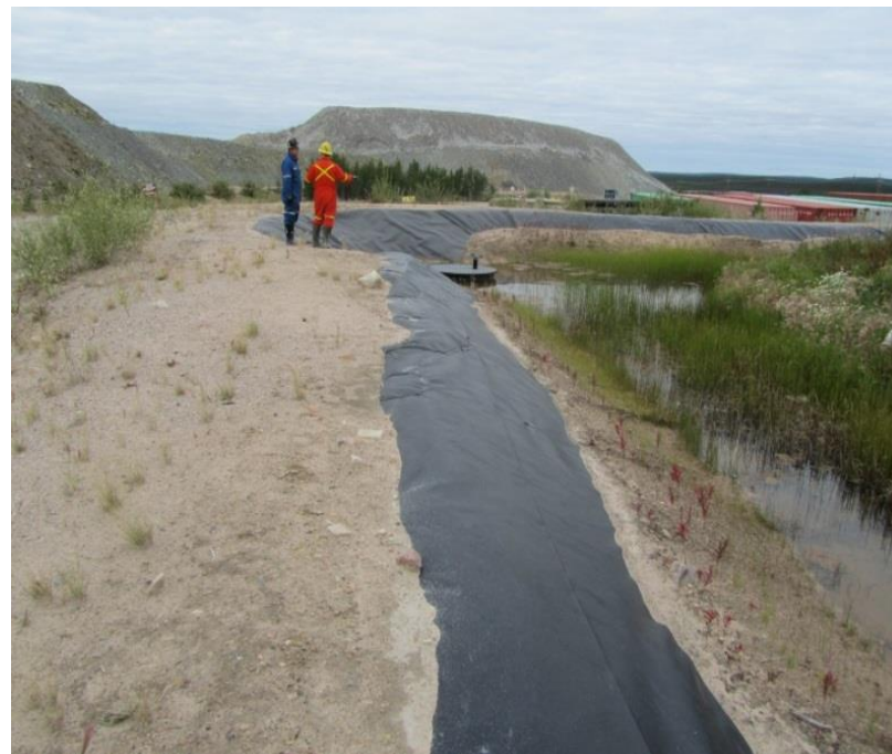
CNSC staff checking berm and ditch conditions – Waste Rock Stockpile B (Photo source: CNSC )
