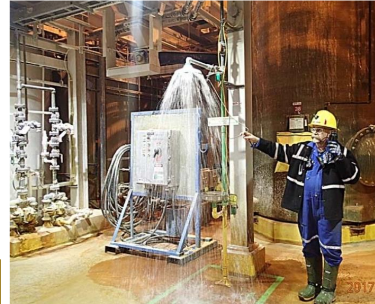
Emergency shower area (Photo source: CNSC)
