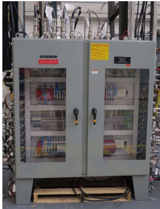
Figure 16 - Electrical Panel to Support Mo-99 IIS Operation
