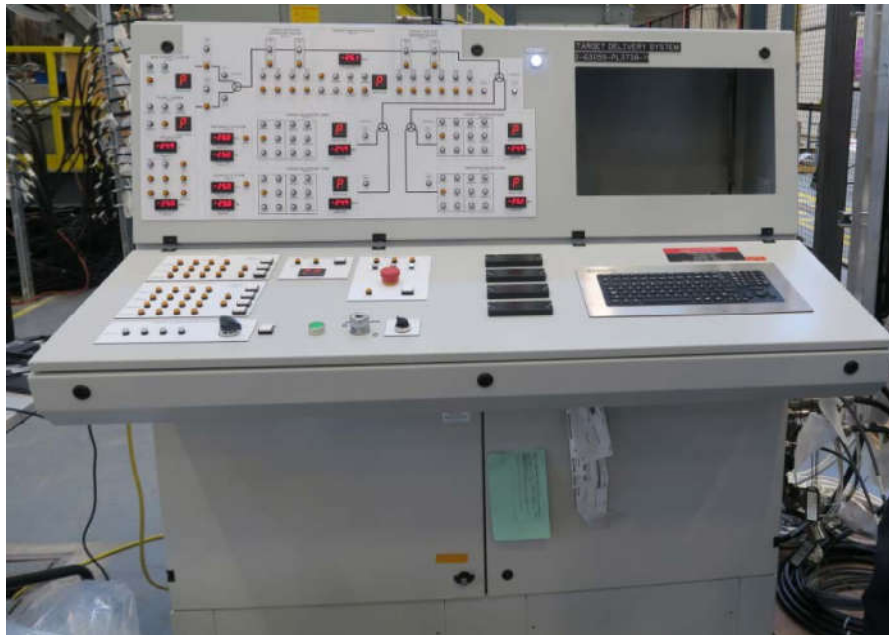
Figure 15 - Mo-99 IIS Local Control Panel
