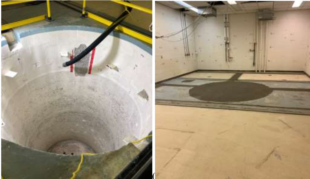
Picture 2: Reactor pool ready for grouting (left) and SRCSF with the pool and overflow channels filled with grout
