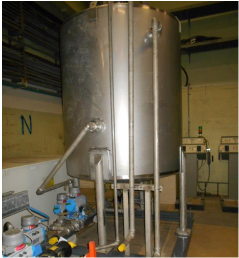
Spent resins removal (ILW)
