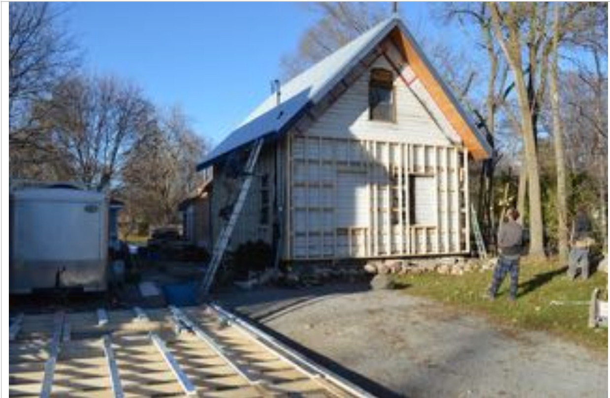
2015 - Framing exterior walls and hanging them off existing framing to add insulation.
