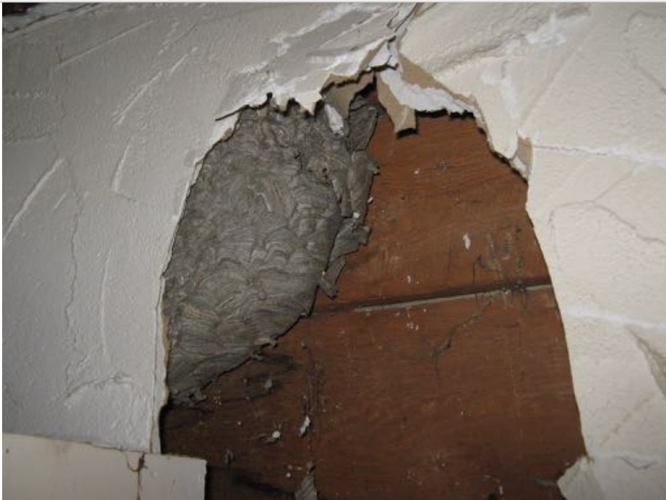
2011 - Wasp nest in the exterior wall
