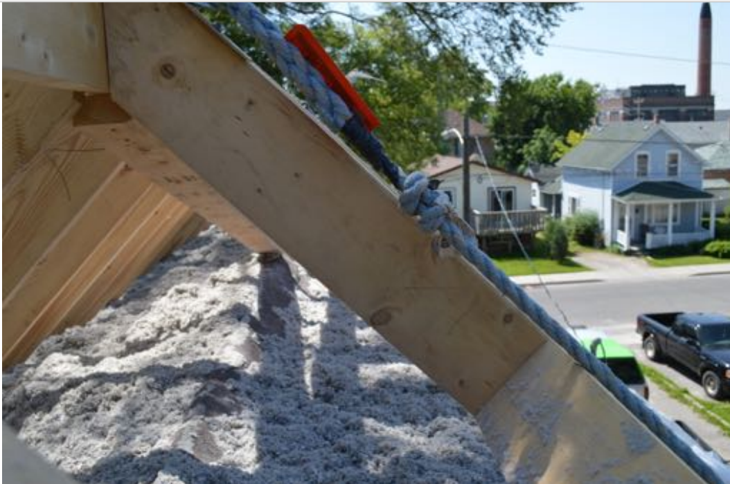
2013 - Framed a new roof over existing as a way of adding 24" of cellulose insulation (R-80)
