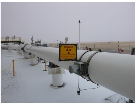
Figure 14: Fixed gauge attached to a pipe (source: CNSC)
