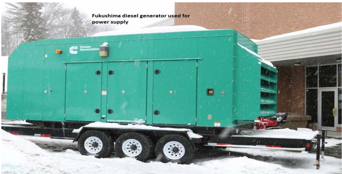
Figure 4: Fukushima Diesel Generator
