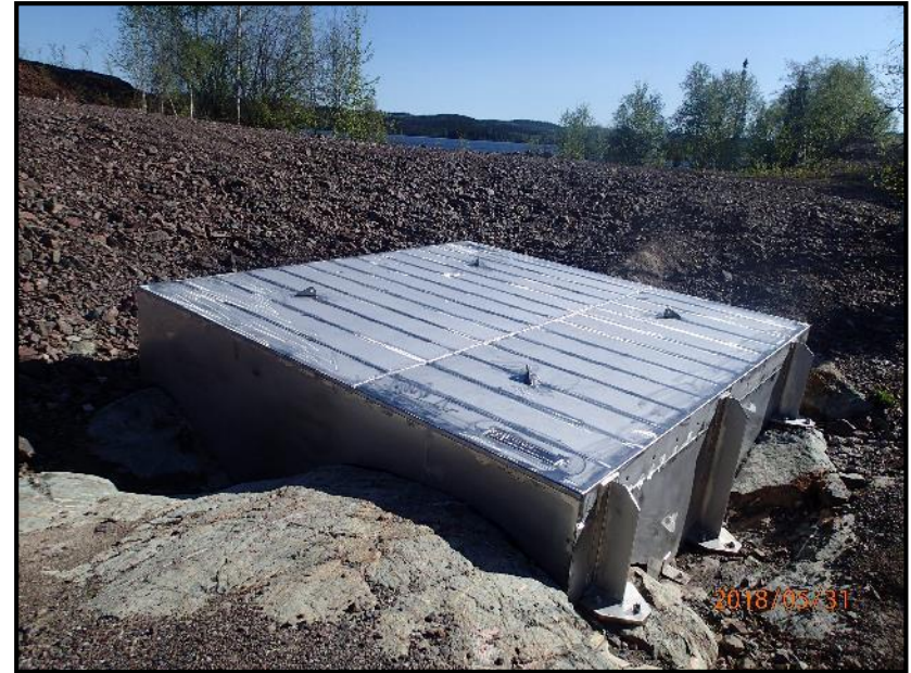
Ace 130 raise cap installed in 2017 (CNSC May 2018)
