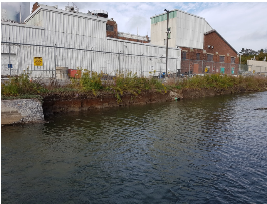
Figure 3: Photograph of collapsed section of harbour wall (view from South)
