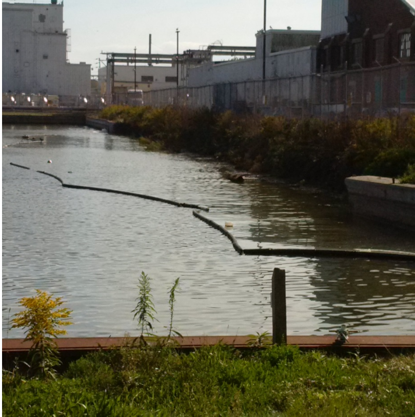
Figure 2: Photograph of collapsed section of harbour wall and silt curtain (view from North)
