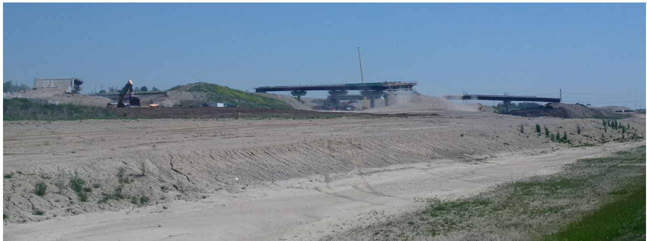
Figure 10: Completed 401/Holt Road Interchange (Top) looking North Along Holt Road from the Darlington Nuclear Site, and East Link (418)/401 Interchange Construction Progress North and West of Darlington Nuclear Site (Bottom)
