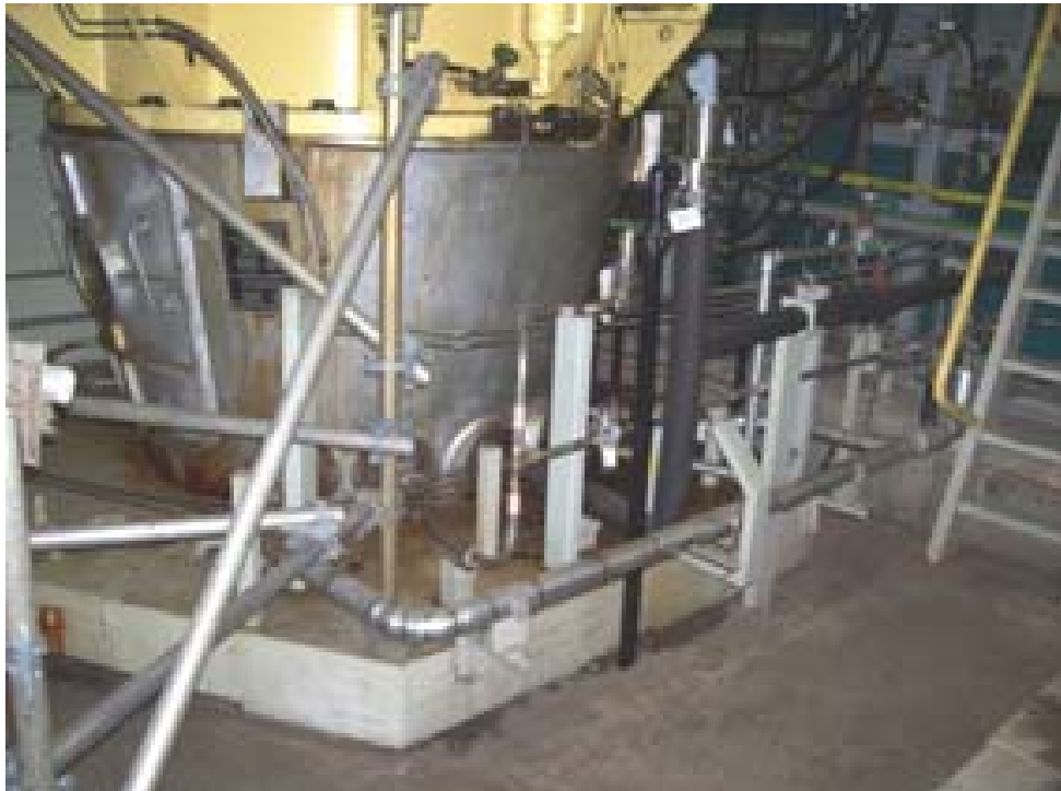
Figure 1: Primary Heat Transport Pump Stool
