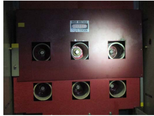
Figure 16: Photo showing circuit breaker with shutter open. Employee was injured in March 2017 when contact was made with top right bus stab.
