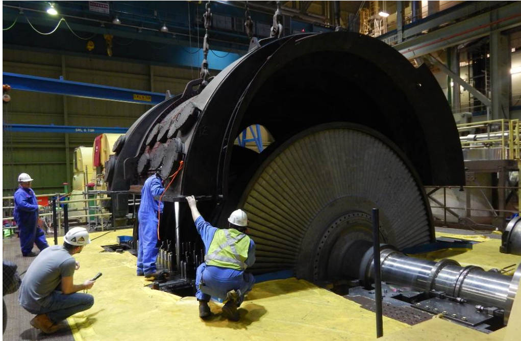
Figure 6: Turbine casing being installed during an unit outage ( photo courtesy of Bruce Power )
