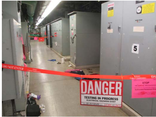
Figure 15: Photo showing work area as left after worker injury in March 2017.
