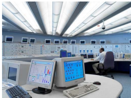
Sizewell B Control Room, Copyright of EDF Energy
