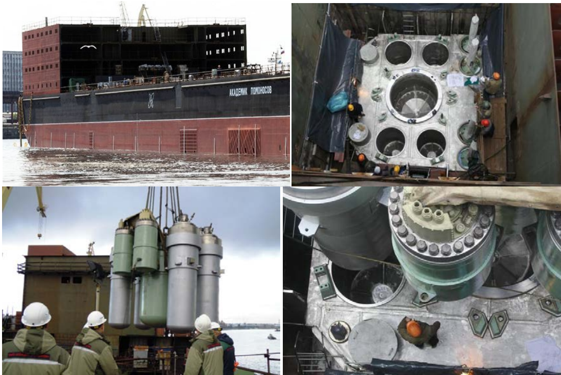
Figure 3 KLT-40S reactor plant unit are being loaded to the floating nuclear power plant (FNPP) 24,25
