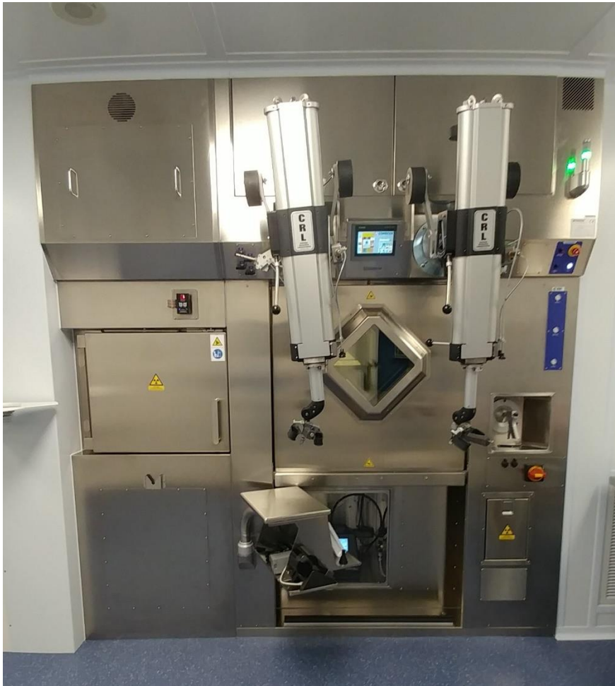
Both hot cells shown have 7.5 cm lead shielding in the walls, floor and ceiling. The lead glass windows are 18 cm thick and have a lead equivalence of 7.5 cm (courtesy of UOHI)
