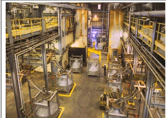
The interior of the Blind River Refinery in Blind River, ON.
