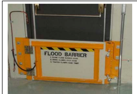
A recently installed flood barrier at Darlington Nuclear Generating Station.
