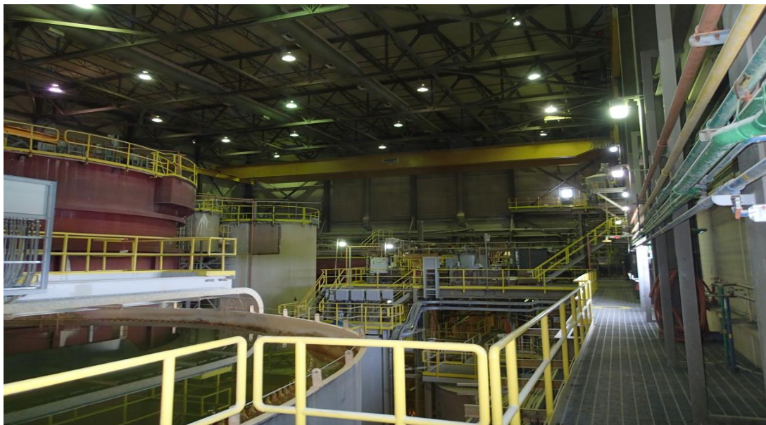
Figure 6-5: Key Lake operation – effluent water treatment plant
