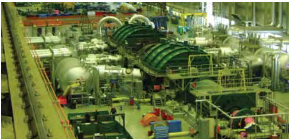
Darlington NPP turbine hall.
