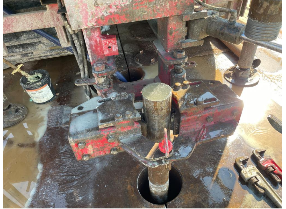
Photo 6: Water in the casing after attempted flushing.
