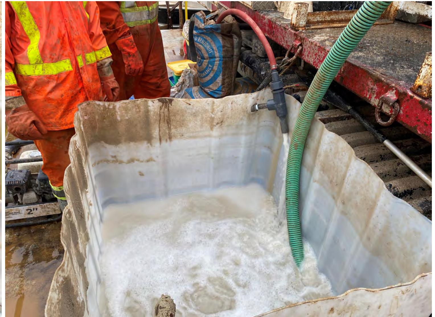
Photo 4: Tank and mixing procedure set-up
