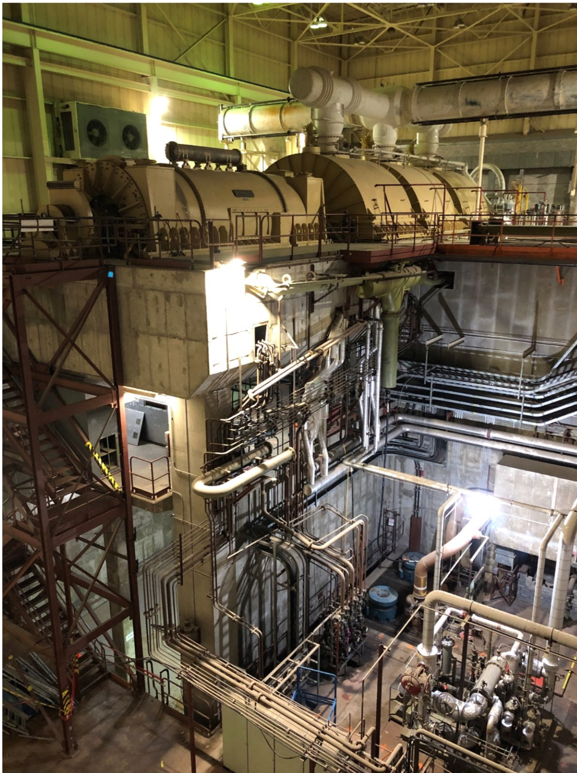
Figure 16: Turbine Building - High Pressure Turbine System
