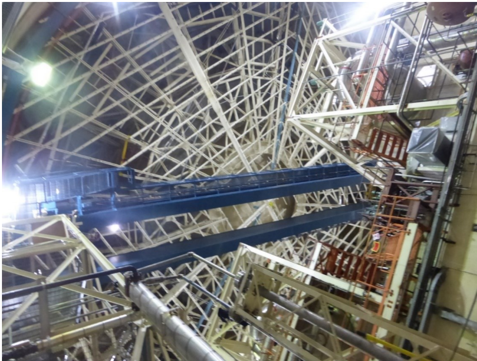
Figure 9: G1WF Reactor Building - Polar Crane and Dousing Tank (above the white structure)
