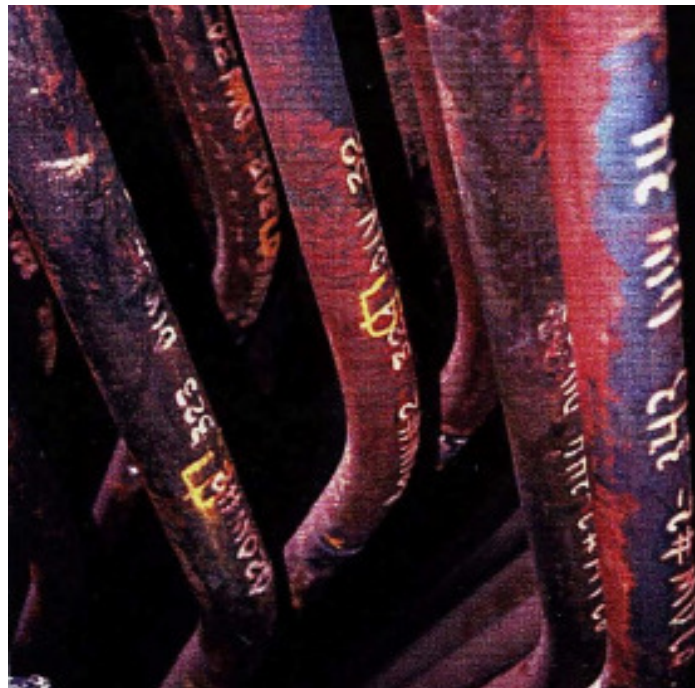
Figure 1 : Feeders oxidized inside a feeder cabinet at Bruce CANDU
