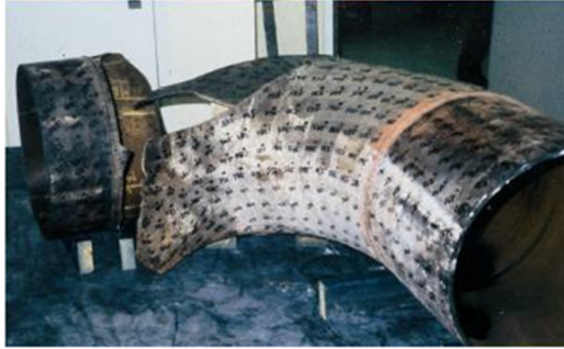
18" elbow wall thickness decreased from 12.7 to 1.5 mm on feed-water pump inlet at Surry, 1986
