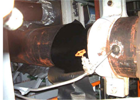
Wall Thickness reduced from 10 to 1.5 mm on Feed-water piping at Mihama unit 3, 2004
