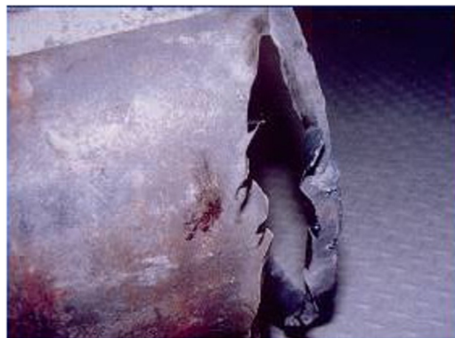
Failure of 14" heater drain extraction line to high pressure heater at Arkansas unit 2, 1986
