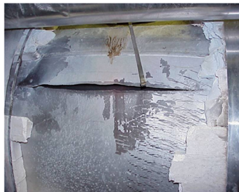
Failure of the Feed-water Heater Point Beach Unit 1, 1999
