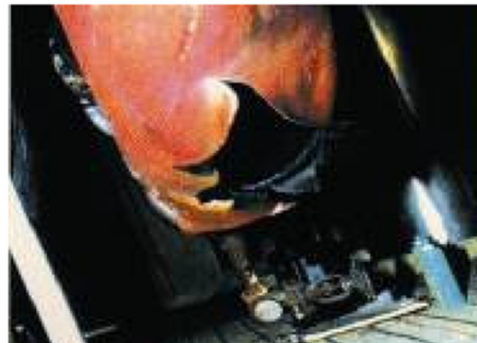
Failure downstream of the LCV in the reheater drain line at Millstone unit 2, 1991.
