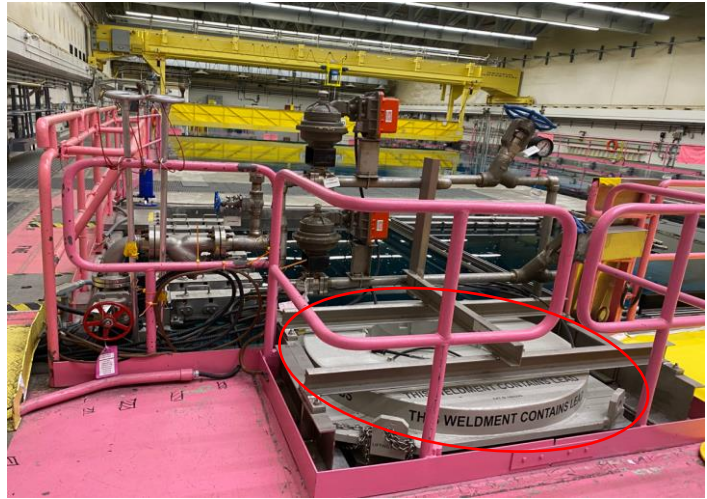
Existing Discharge Equipment (Removable Flask Platform Shown in Red)
