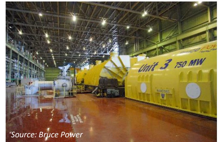
Bruce NGS A turbine interior
