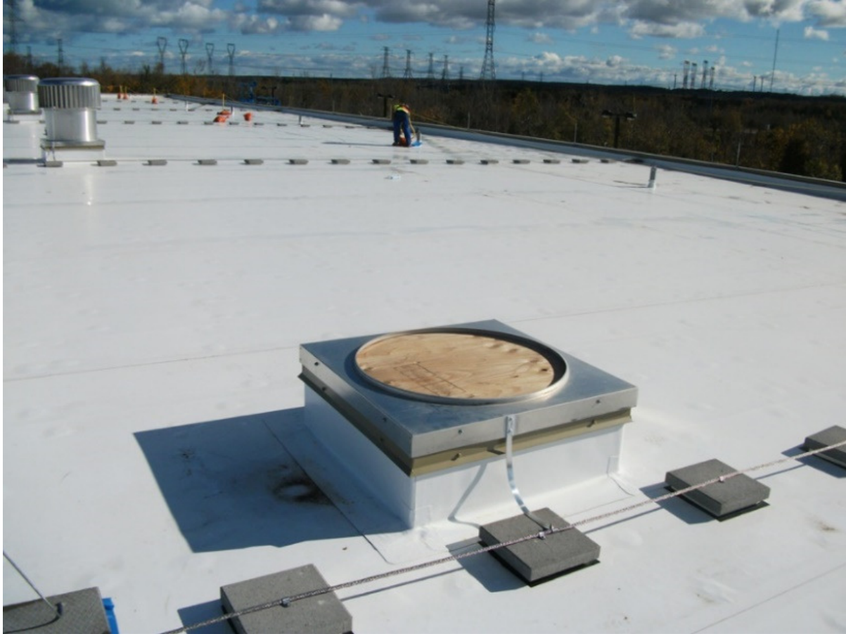
Figure 8: Top of OPG western waste management facility in Tiverton, ON – installation of storage building ventilations that discharge unfiltered air from DSC storage building (Source NAENG.COM)
