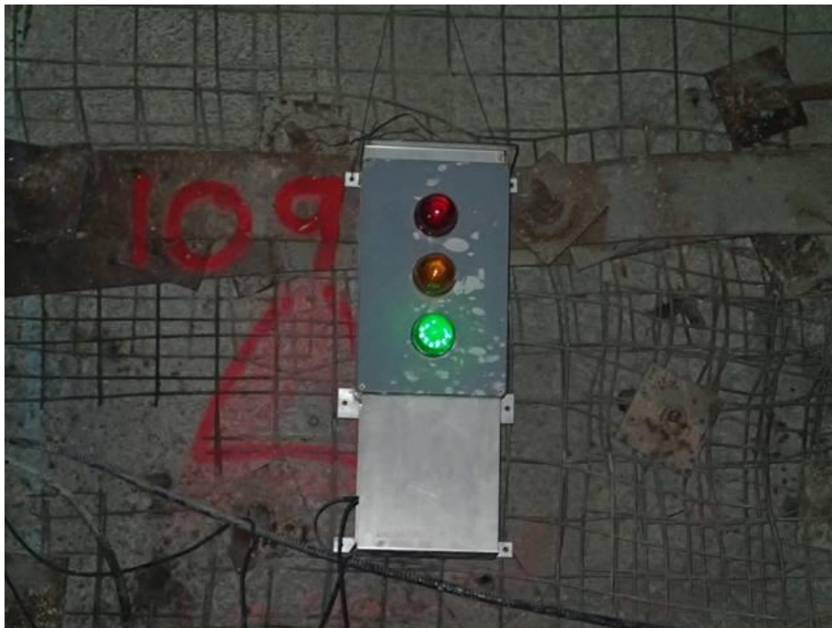
Figure 2.4: alphaNUCLEAR PRISM at an underground mine
