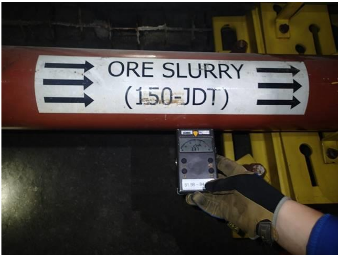
Figure 2.3: CNSC staff measuring gamma dose rate on ore slurry pipe
