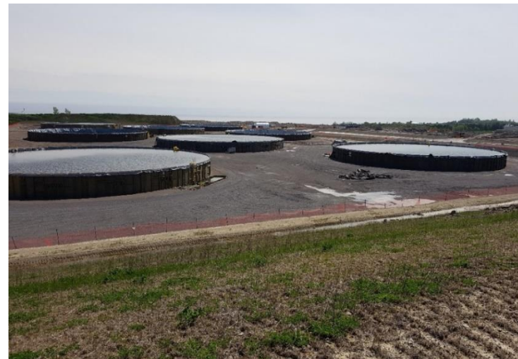
Lake Tanks used for Additional Water Storage at the PGP, a project to remediate legacy contamination in the Municipality of Clarington
