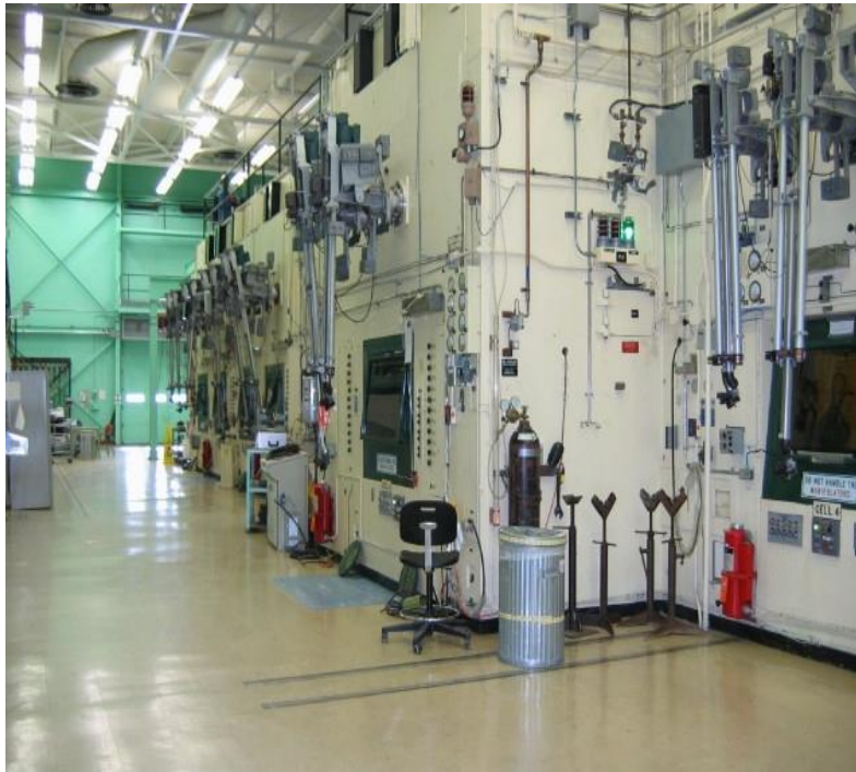
Figure 3-17 : HCF Operating Area South View (Rooms 1-82/1-83 and Cells 1 to 4 (left to right))
