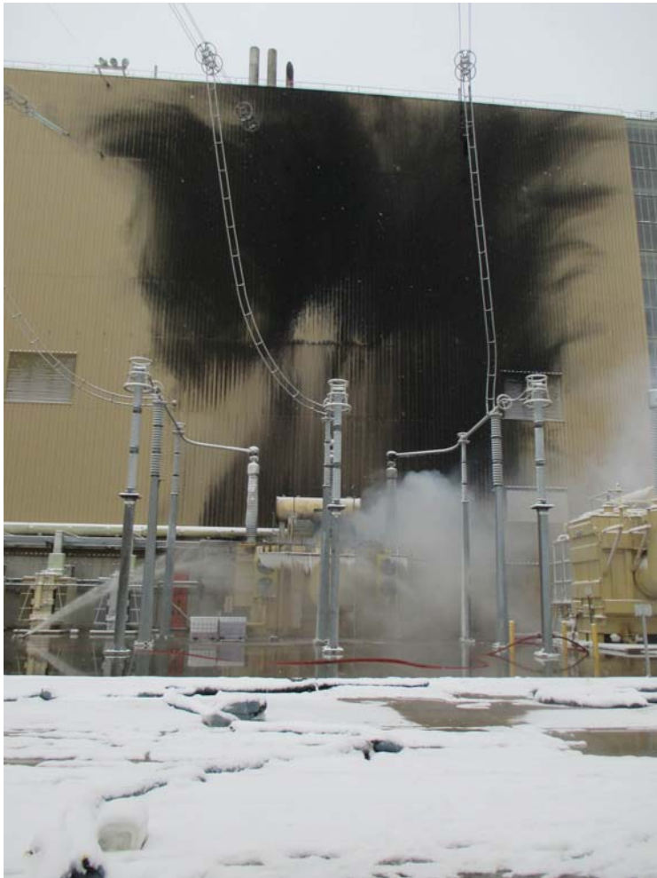
Figure 4: Photograph of Transformer and Powerhouse Wall on Dec. 7, 2018 after the Fire was Extinguished
