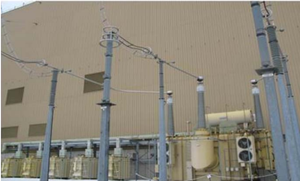
Figure 3: Photograph of a Station Service Transformer at the Bruce site
