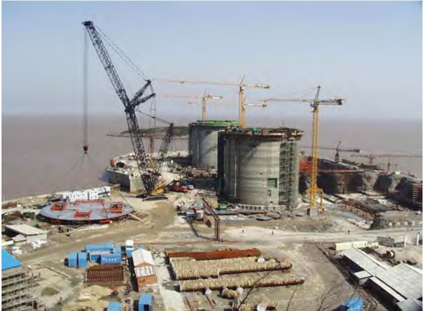
Construction of CANDU-6 Nuclear Power Plant at Qinshan, China using Liebherr LR1600/175- Very Heavy Lift Crane (Rixin and Petrunik 2003)
