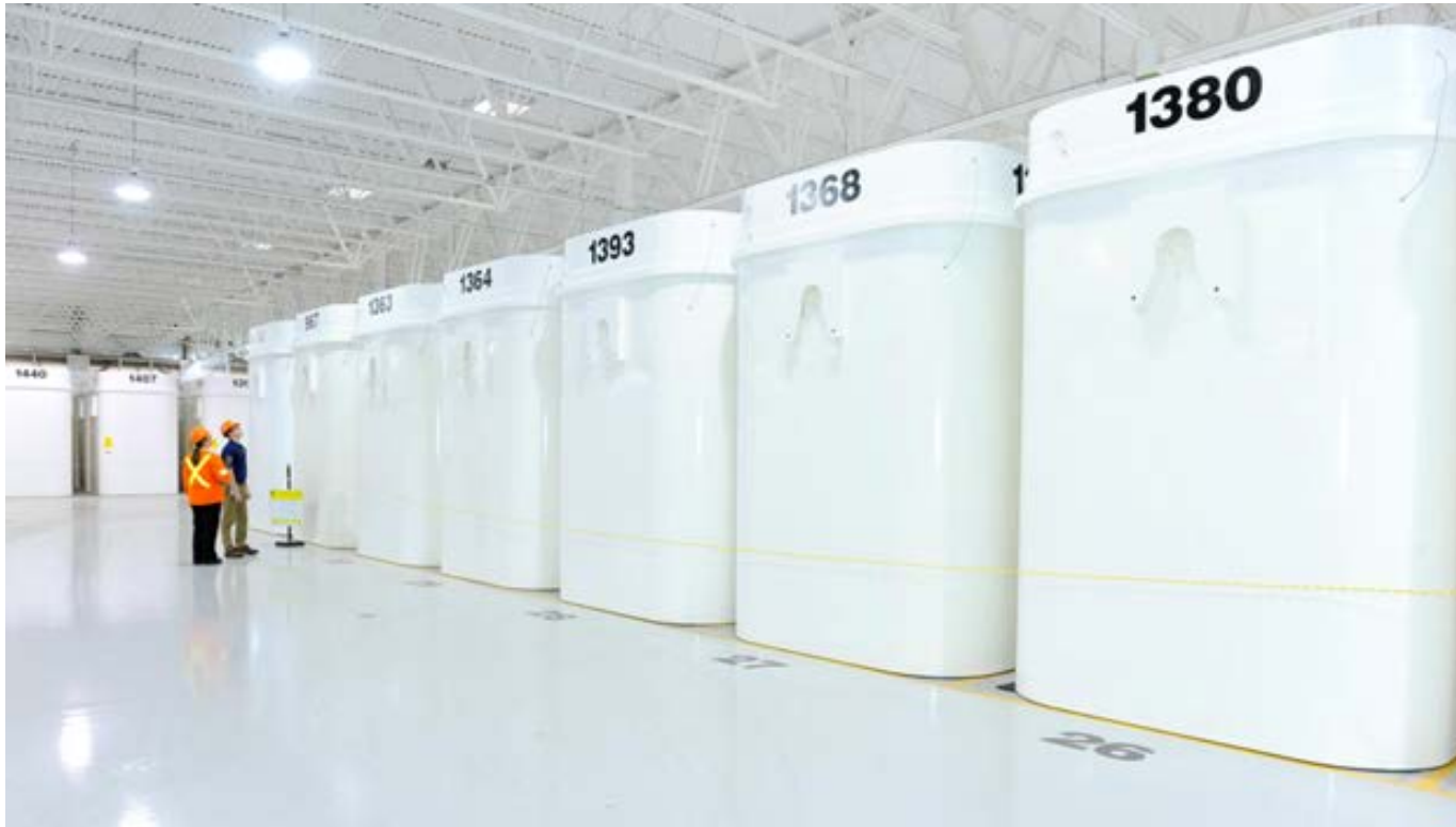
OPG used fuel dry storage containers at the Western Waste Management Facility
