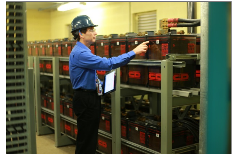
Battery Bank, Bruce Nuclear Generating Station
