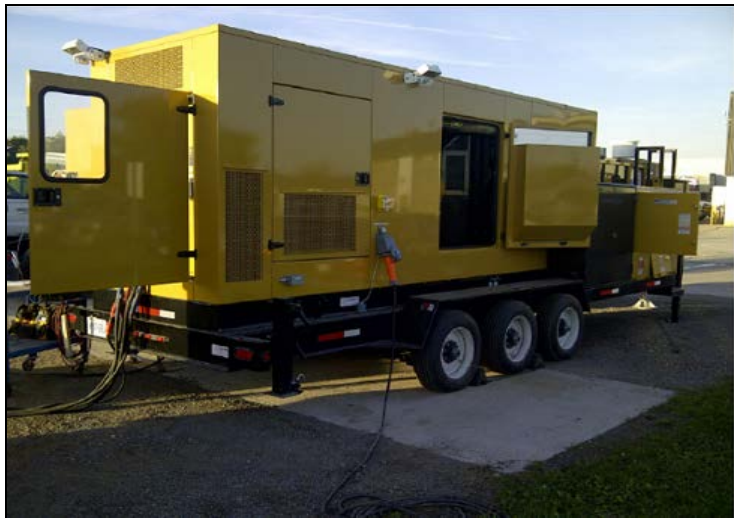
Bruce A 400 kW Generator (2)
