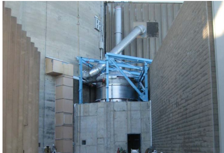
Containment filtered venting at Point Lepreau
