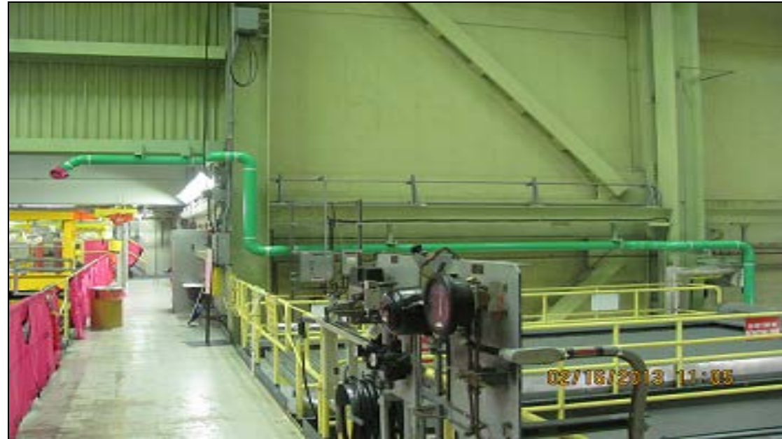
Permanent piping to spent fuel pool
