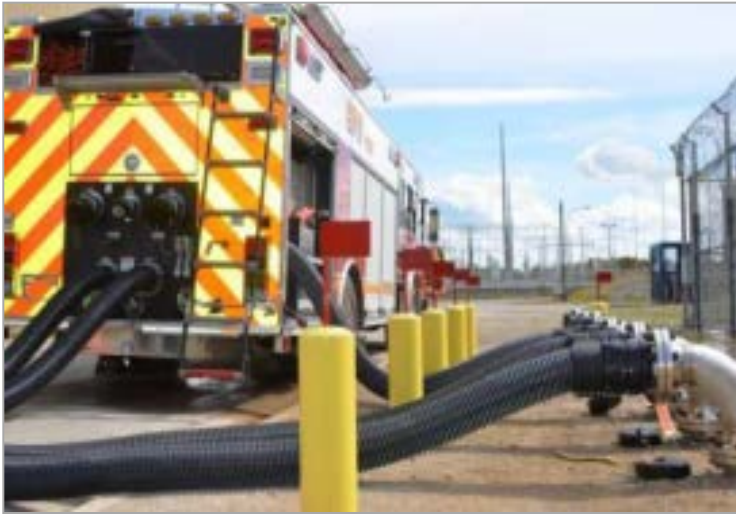
Bruce Power fire trucks provide cooling water. New emergency water pumping equipment procured and on site
