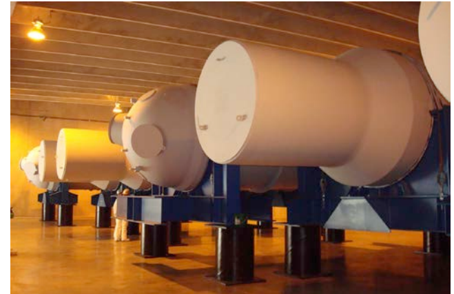
Steam Generators in safe storage state. Photo courtesy Bruce Power.
