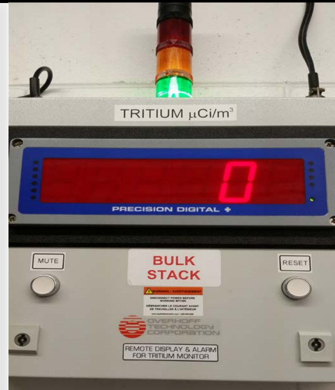
Bulk stack real time display with visual and audible alarm.
