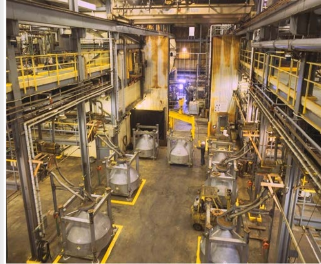
UO_3 tote bin loading and handling station at the Blind River Refinery.
