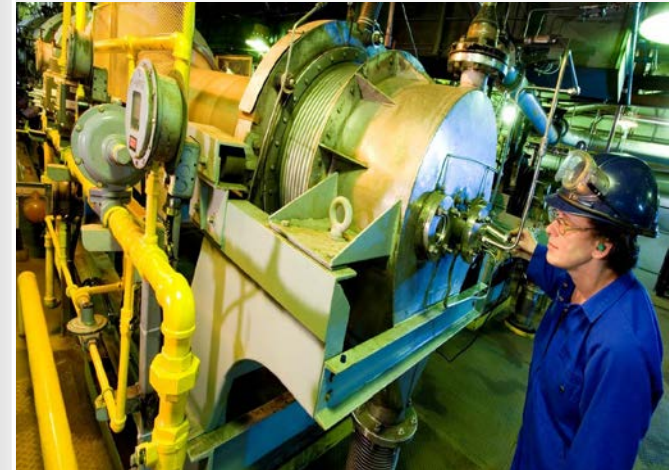
Port Hope Conversion Facility worker performing visual check on \text{UO}_2 inside rotary kiln.
