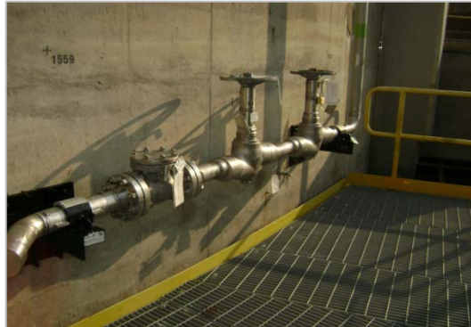
Point Lepreau, calandria vault make-up
