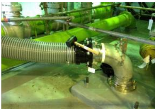
Point Lepreau connections to emergency water supply, freshwater pumphouse
