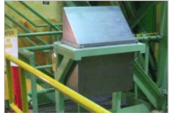
Hydrogen control and mitigation with licensees have enhanced hydrogen control through installation of PARs.
