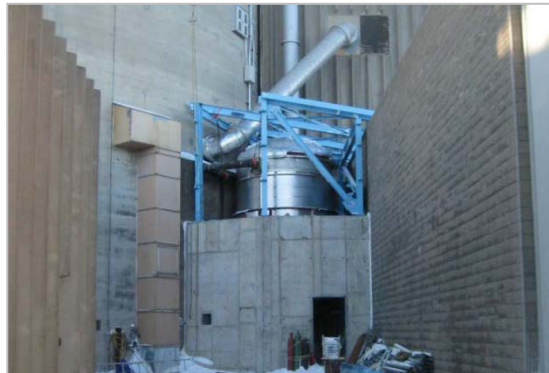
Containment emergency filter venting system
