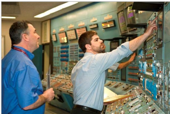
Control room operator reviews emergency operating procedures.
