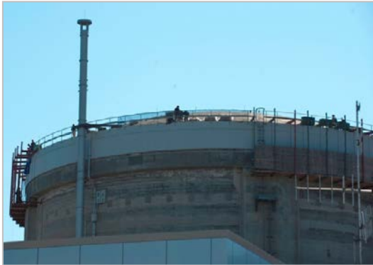
Point Lepreau emergency filtered vent stack
