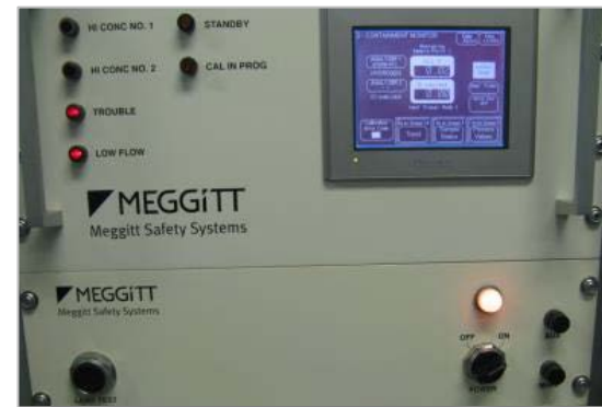
Severe accident sampling and monitoring system
