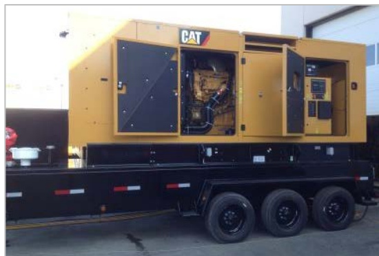
Backup power generator and connections - PLNGS has 4 in total
