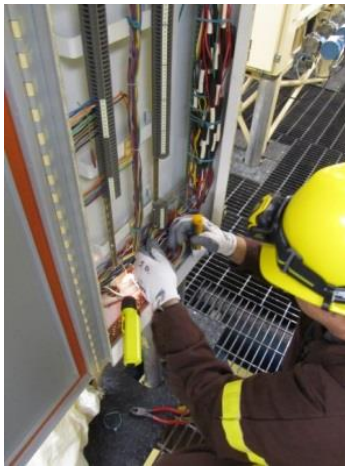
Removal of cable samples from the Gentilly-2 Facilities to be used for verifying initial assumptions. This is one of the locations within the site where samples have been extracted for this study.
